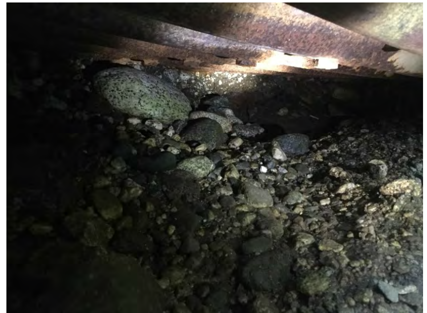
Scour Under Outlet 1
